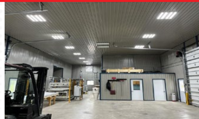
Plastic Extruding Shop Ceiling Mounted (6500K - No Lenses)
