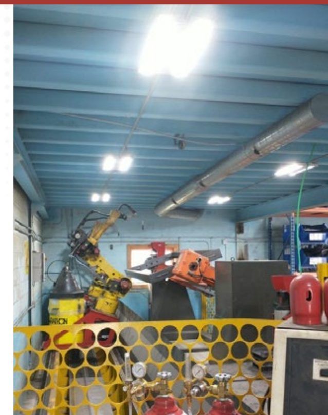
Welding Shop Ceiling Mounted (6500K - No Lenses)
