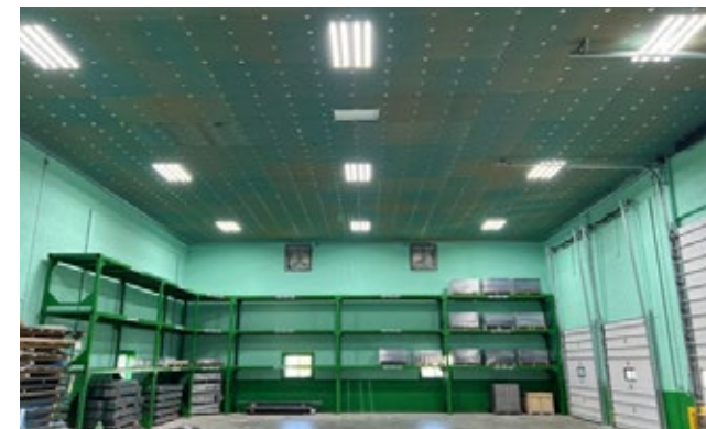
Shipping/Receiving Warehouse Ceiling Mounted (6500K - No Lenses)
